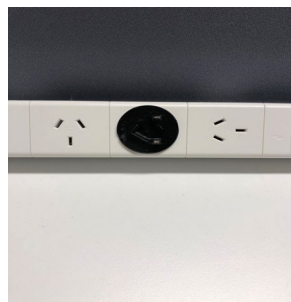
Photo 2: Pins remaining in the power board
