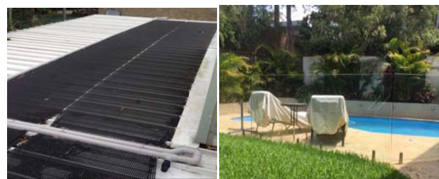
Figure 1 Residential solar pool heating system.
