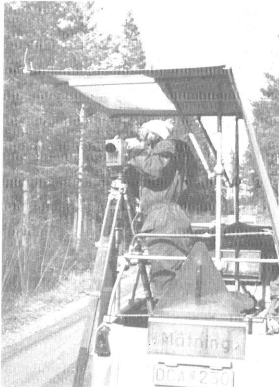
Figure 5.10: Instrument vehicle in motorised precise levelling in Sweden with Zeiss Ni002 (after Becker 1979)
