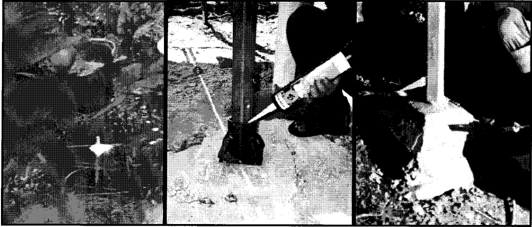
Figure 4.6 - Monuments emplaced on Gunung Papandayan, A) Concrete and reinforcing rod extends to a depth of 1-metre, B) the fiberglass rod is braced with a steel mount, C) final concreting around the base of the monument.
