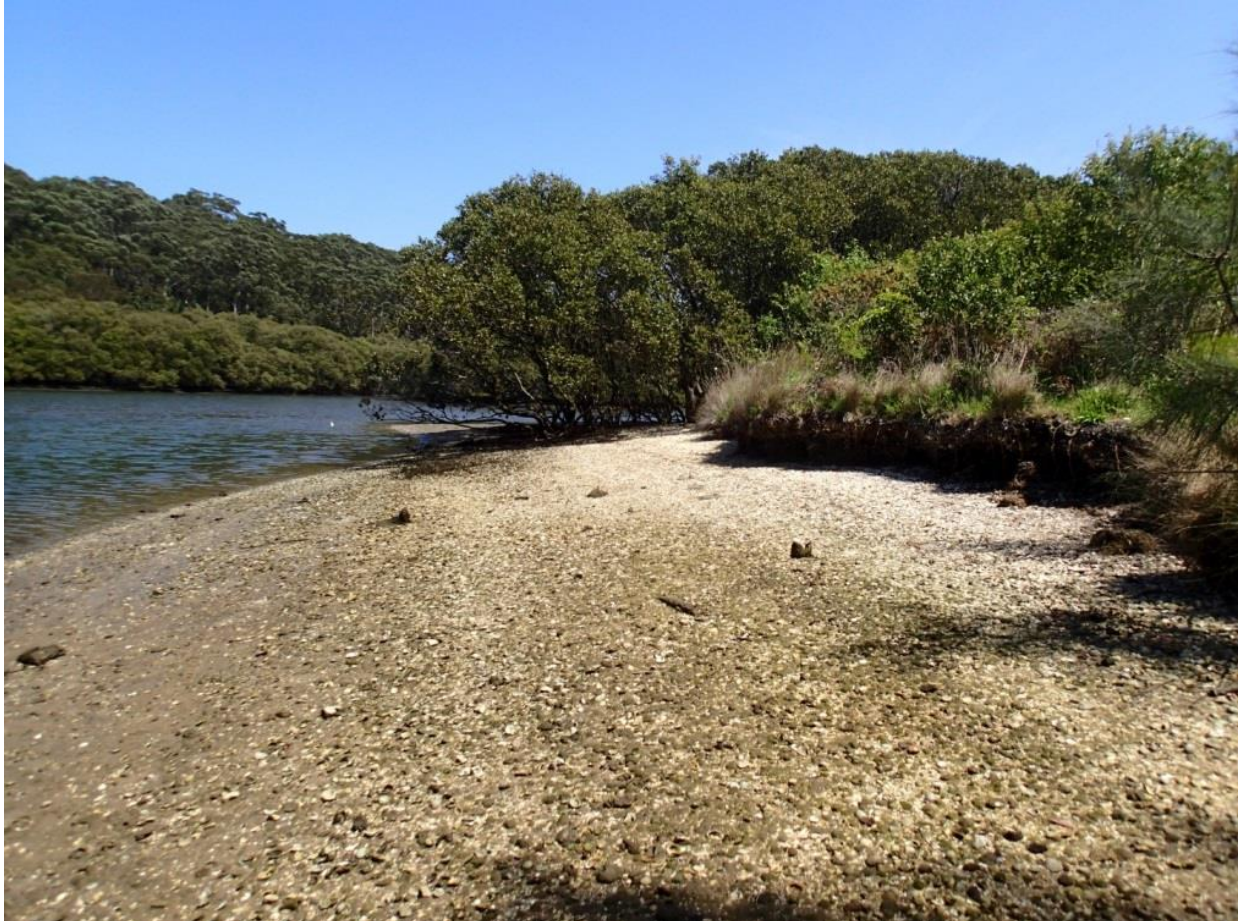
Figure 2-1: Example Proposed Field Site Experiencing Bank Erosion for Oyster Shell Bag Structure Sugarloaf Point (Lane Cove River National Park), East Ryde
