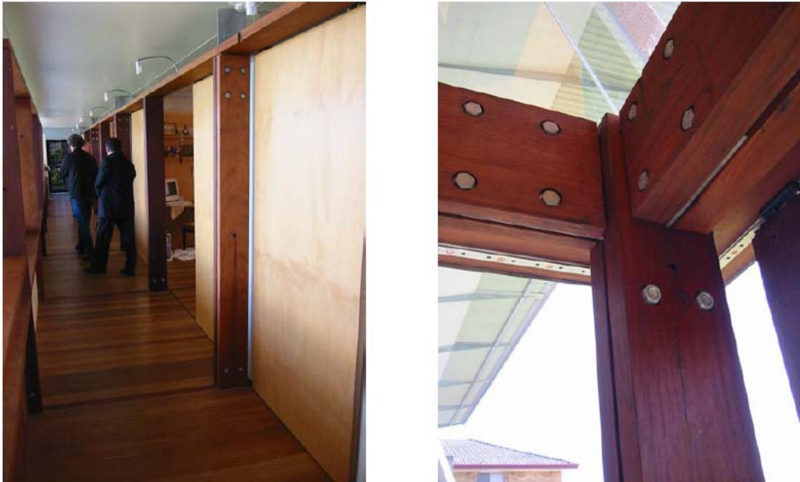
Figure 2: An example of a modular design and detailing for deconstruction (Graham 2005, p. 7)
