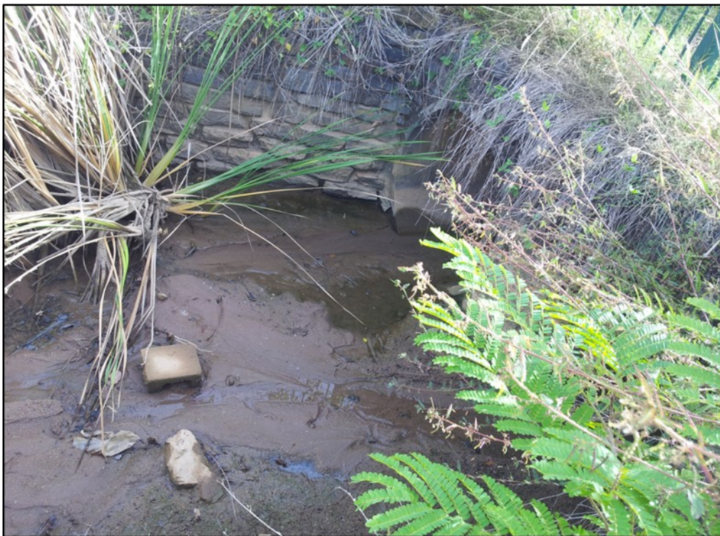
Inlet Zone at Fairway Waters in Durack Illustrating the High Sediment Loading of Incoming Waters
