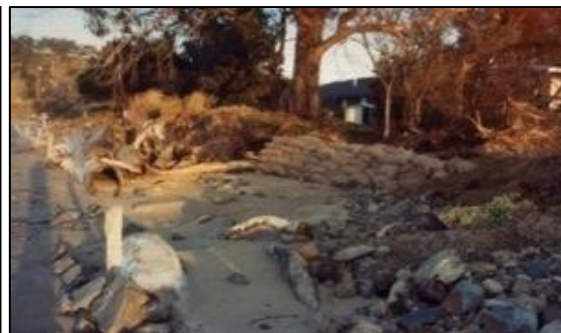
Image 3: Erosion on the end of a rock wall, Roches Beach - City of Clarence 2010
