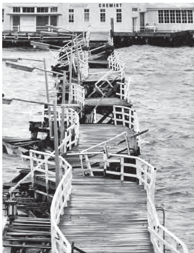
Storm damage to Manly promenade, Sydney 1974.
