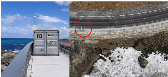
Figure 5 Camera installed at Ōhau Point (circled)
