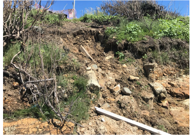
Figure 4 Eroding embankment unearthing artefacts
