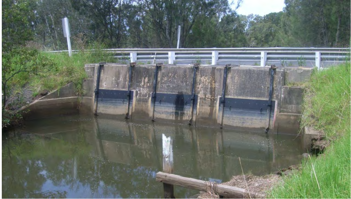
Figure 2-1: P10G1 Crookhaven River floodgates at Culburra Rd (Photo: S. Nichols/DPI)
