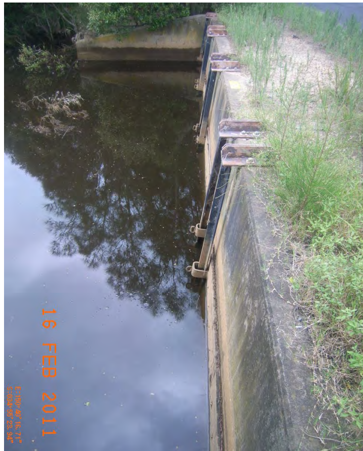
Figure 2-2: P7G1 floodgates at Mayfield Rd (Photo: Shoalhaven City Council)
