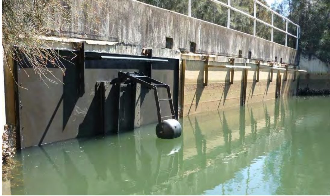
Figure ES.1: Example of a buoyancy controlled auto-tidal floodgate installed on a similar structure (Photo: S. Nichols/DPI)
