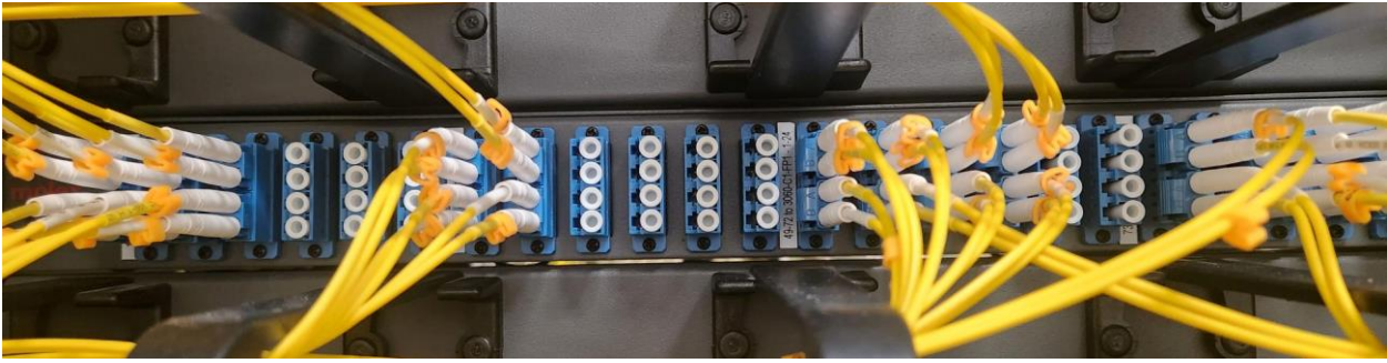
Image 1 - 96-core high density fibre optic breakout tray in a Building Distributor cabinet
