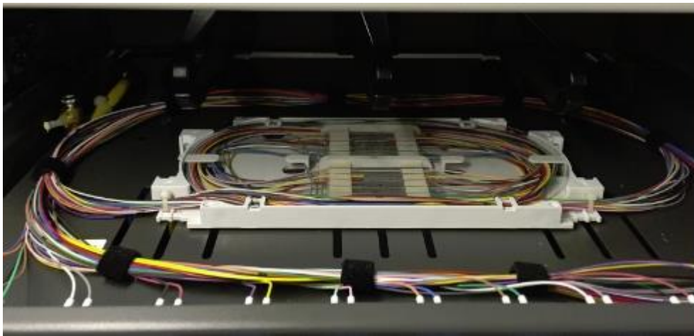
Image 2 - 48-Core Fibre Optic Breakout tray in a Floor Distributor cabinet
