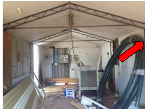
Figure 4: Fowlers Gap Field Station, Generator Shed, Ground Level, Walls and Ceiling Throughout – Fibre Cement Sheeting
