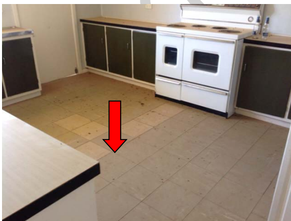
Figure 5: Hay Field Station, Building HFS7, Ground Level, Room G07 - asbestos containing vinyl floor tiles
