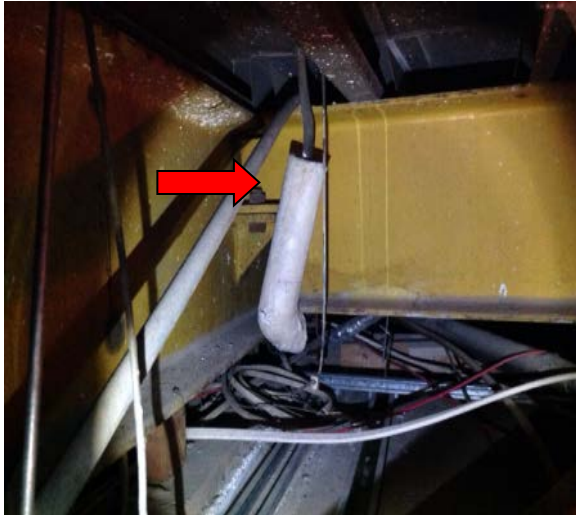
Figure 13: Kensington Campus, E6 Roundhouse, Ground Level, Room GQ14, ceiling space pipework insulation, lagging
