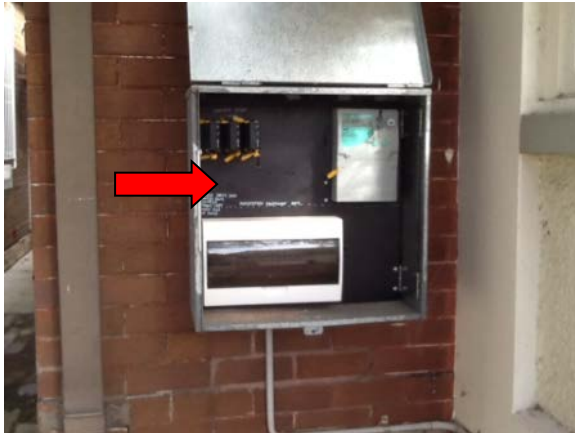
Figure 7: Kensington Environs, 32 Botany Street, Ground Level, Exterior South-East Side, Switchboard – Compressed bituminous electrical panel
