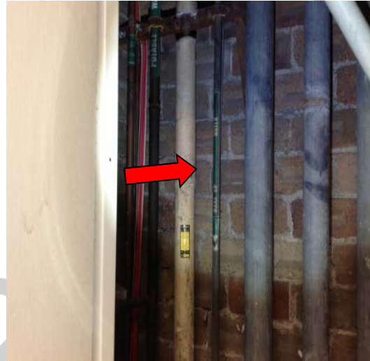
Figure 14: Kensington Campus, K15 Old Main Building, ground Level, room G69A duct – pipework insulation, lagging
