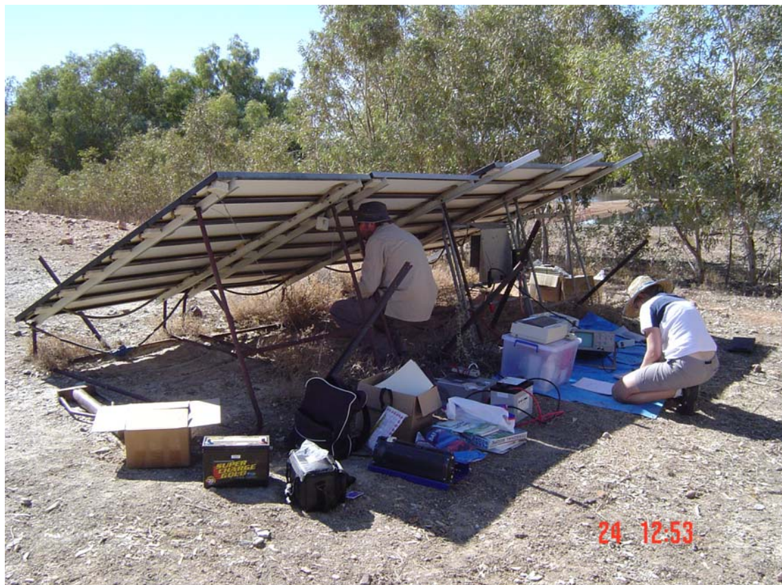
Fig. 1. Shelley Bambrook and David Croft diagnose the Freislich Dam solar powered pumping system.
