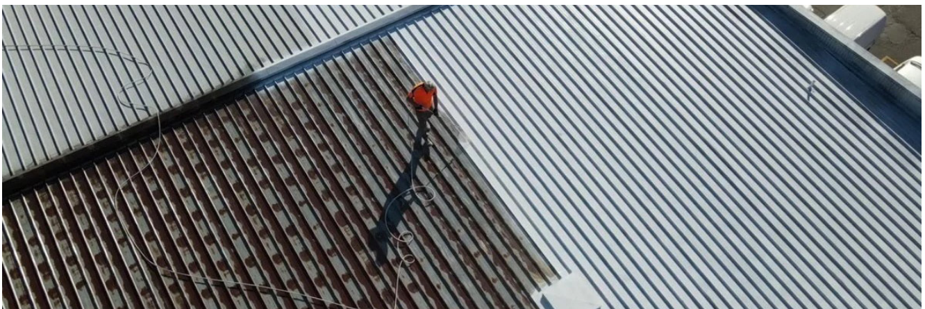
Figure 2.10 Example of a field-applied cool roof coating on a commercial building in Victoria (source: energystar.com.au ). The application of a cool roof coating also improves the resistance to corrosion.
