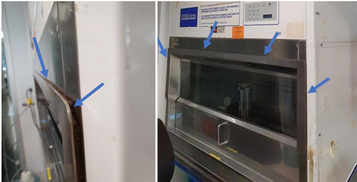
Photo 1: Arrows show the location of air leaks
